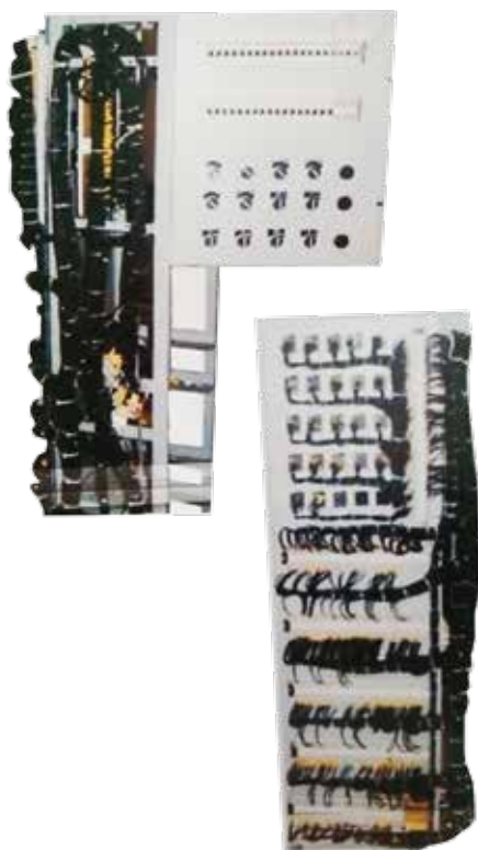
Painéis auxiliares embarcados Panel on board
